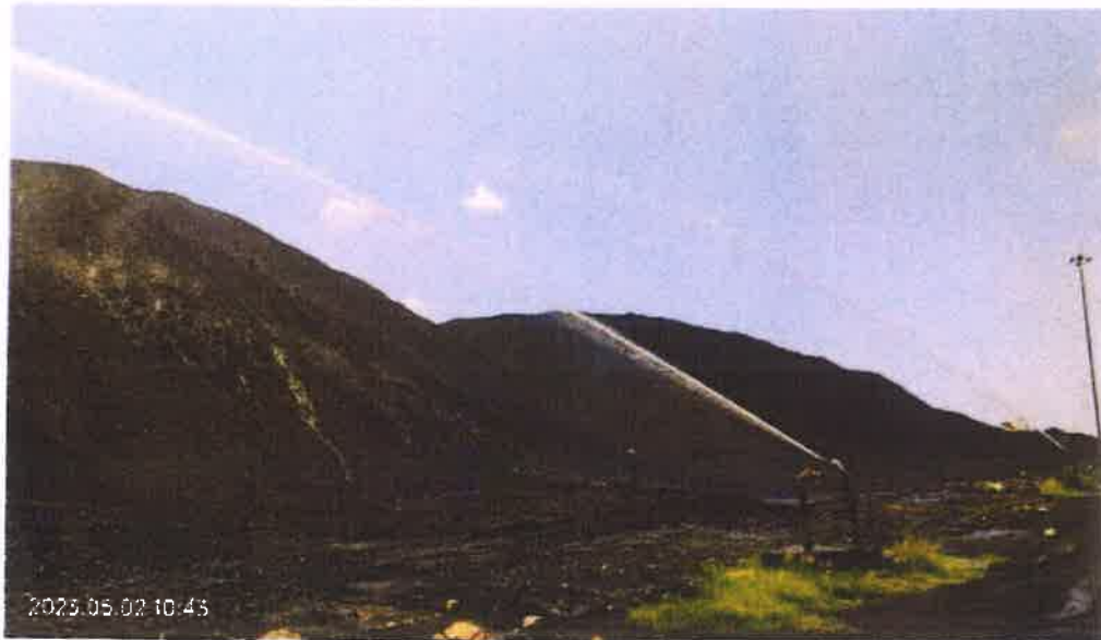
Dust suppression system installed at coal yard
