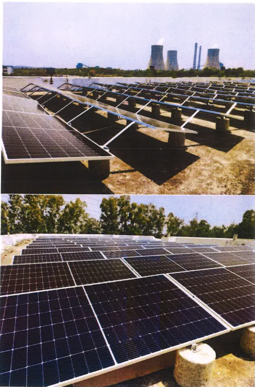
Roof Top Solar Installed at Hospital Building
