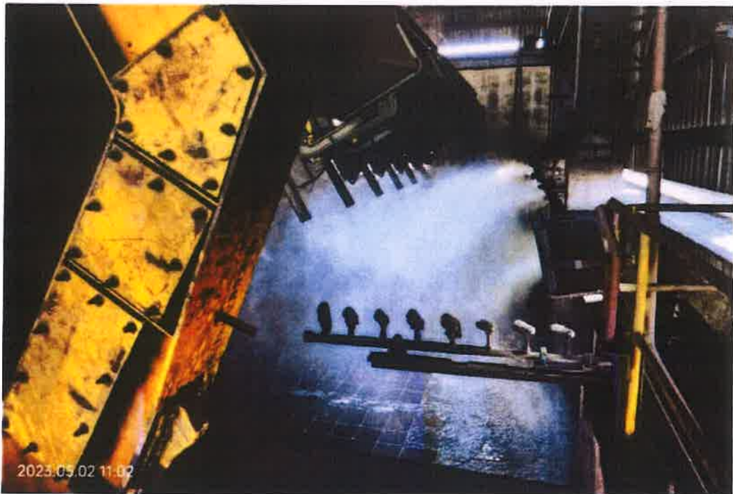
Fogging system at wagon tippler area
