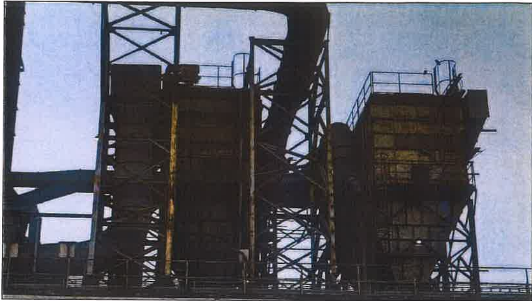
Bag filter installed for particulate emission control
