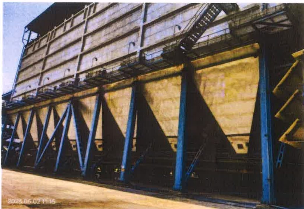
ESP installed for particulate emission control
